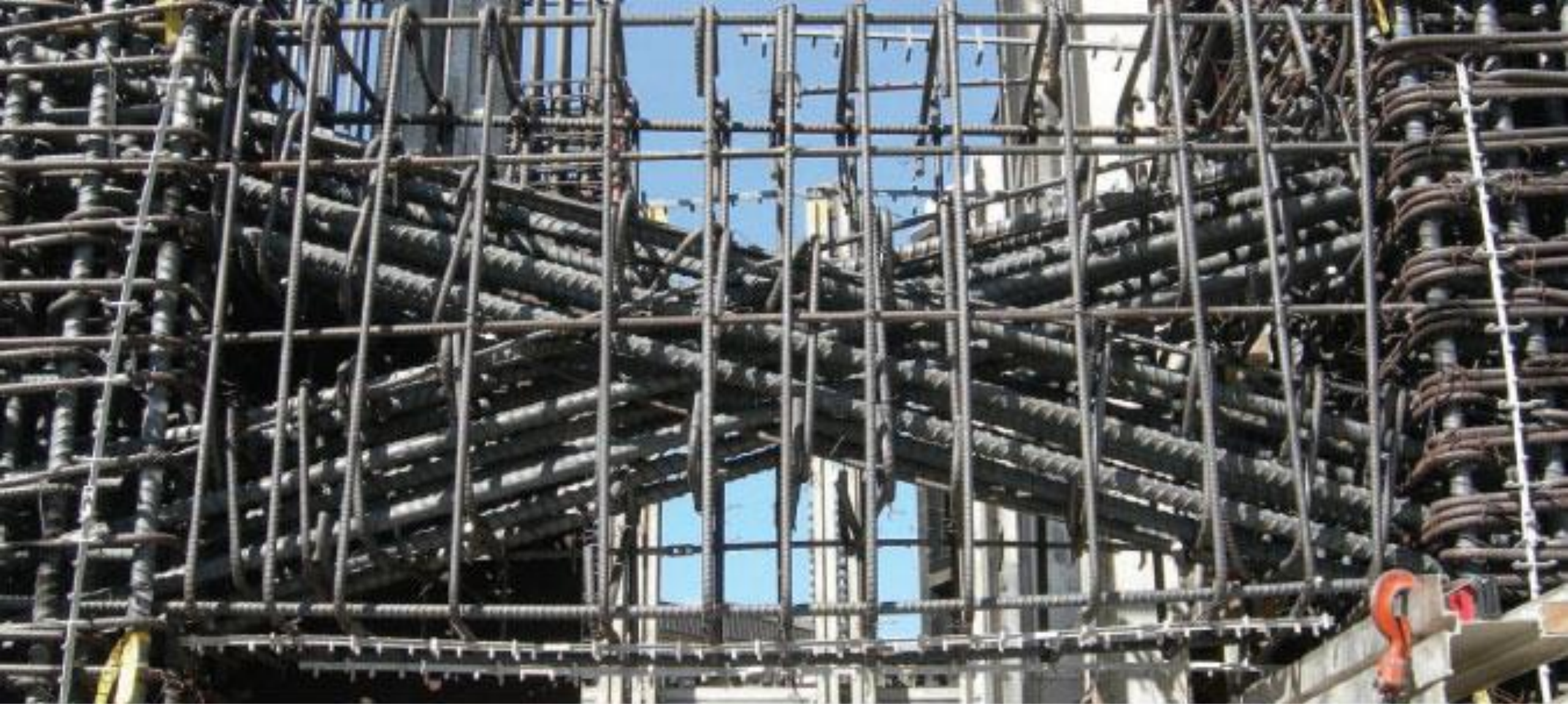
Figure 1 Showing the intricate, labor-intensive steel reinforcing bar congestion in a typical high-rise coupling beam. Photo credit: Remy Lequesne, The University of Michigan
