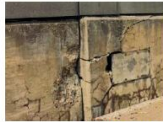
Damage of Wall Deck
