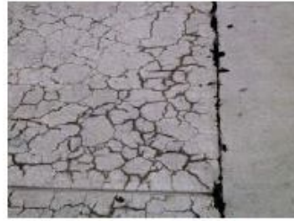
Damage of Asphalt
